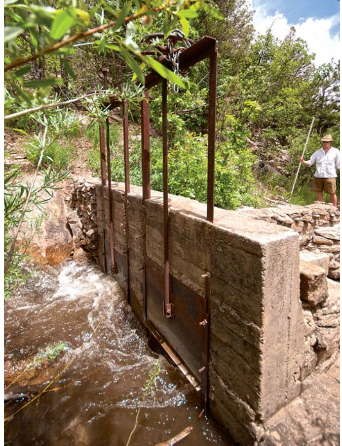
This modern concrete acequia headgate controls the flow of water into fields through multiple “doors.” The local mayordomo decides how to share the water channeled from rivers and streams.
